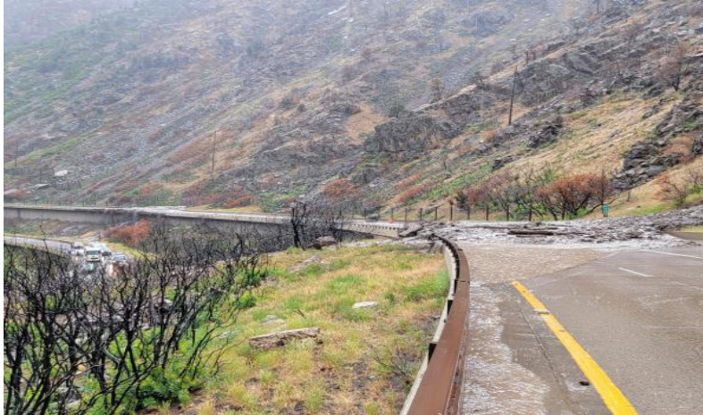
Debris flow covering westbound lane of I-70 5
