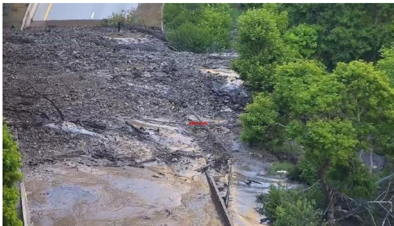
Debris flow covering eastbound lanes of I-70 4
