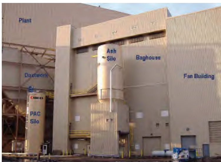
TOXECON™ System Installed at PIPP
