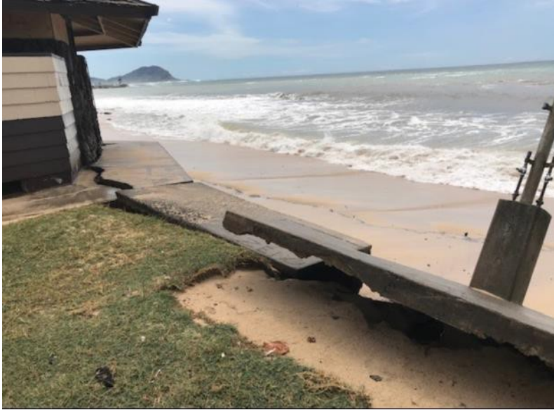
Figure 10: Destruction of Public Facilities, Maunalahilahi Beach Park, 2018
